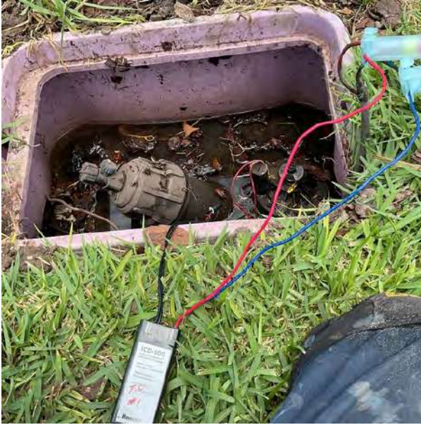
Zone #1 (Valve Status) - 06-09-26 5:38 am CDT
