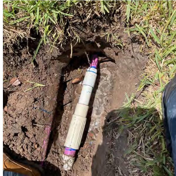
Zone #2 (Broken Lateral) - 06-09-26 5:39 am CDT
