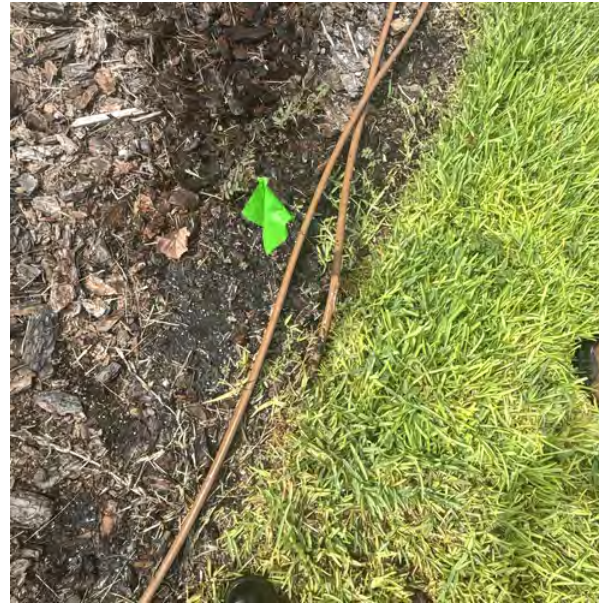
Zone #7 (Broken Drip or Micro Spray) - 06-11-26 9:21 am CDT
